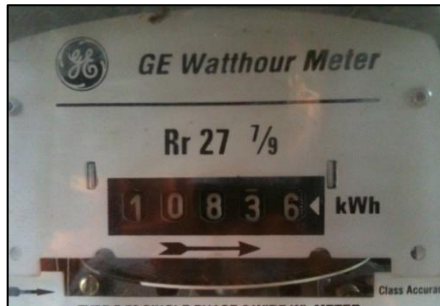
Initial meter reading at 1600 hrs on 20 Feb 2012
