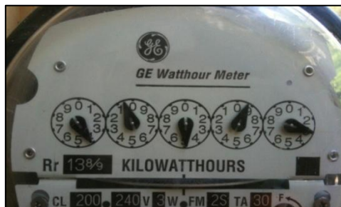
Initial electric meter reading at 0812 hrs on 14 Feb 2012
